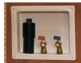
Residential washer/dryer hook-up in laundry closet.
